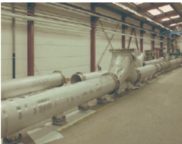
Rohrleitung aus Werkstoff Nr. 1.4435 ø 711,2 x 6,0 mm/ Pre-manufactured pipe spool out of quality 1.4435 (316 L)
